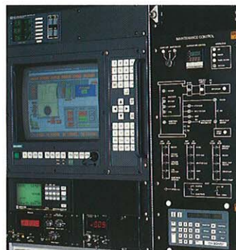
SSC-600 System controls
